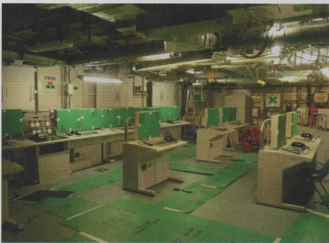
LEFT: When this room is completed it will monitor and control all the ship's systems. BOTTOM LEFT: Captain Ian Groom MBE RN. The engineering specialist who is the master of all he surveys until it goes to sea.
